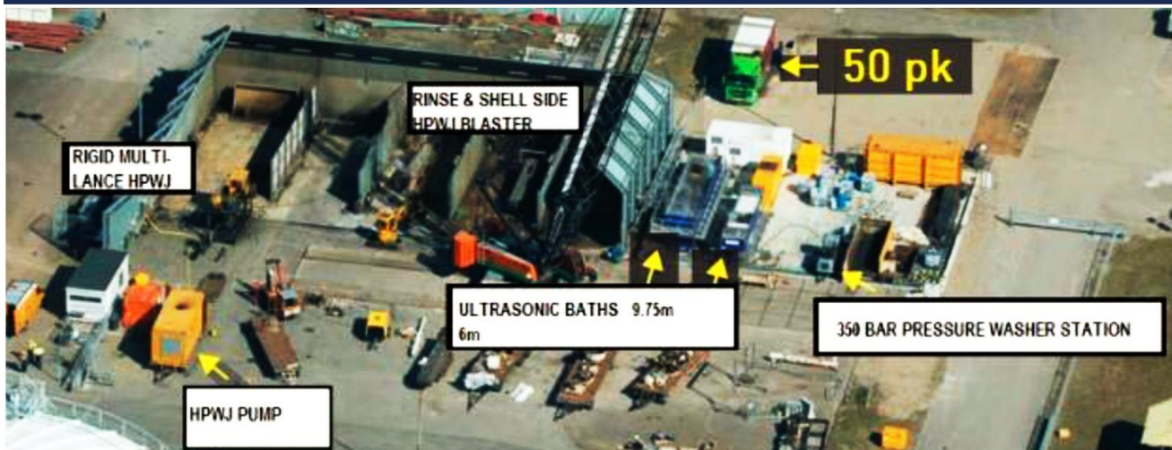
FIG. 3 WASHPAD LAYOUT FOR THE 2013 SHELL MOERDIJK MLO TURNAROUND INCLUDING TWO LARGE ULTRASONIC BATHS
